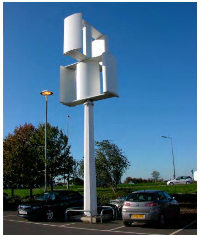
ONSITE WIND TURBINE
